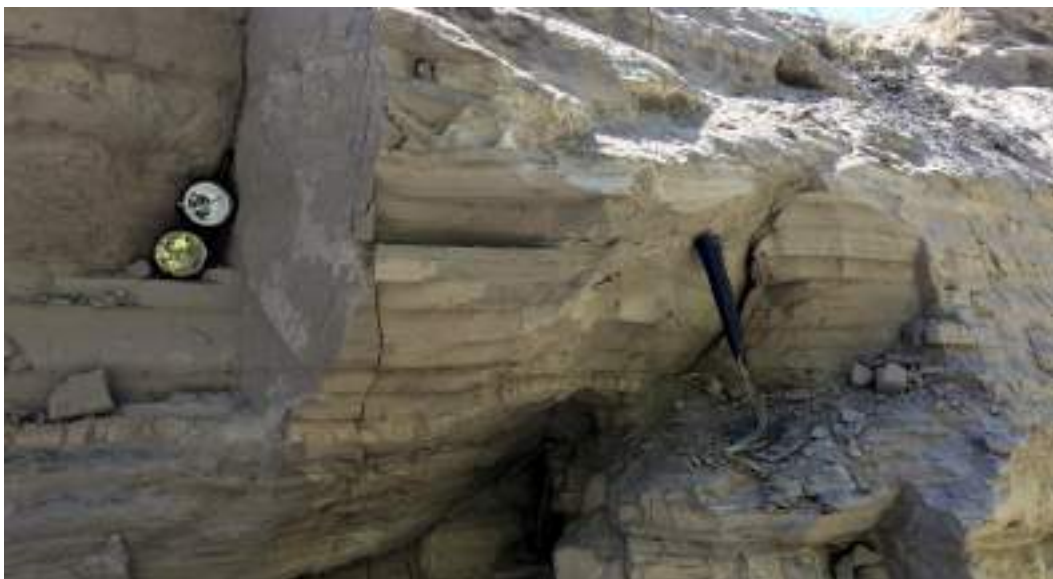
Photo 6-9 View of Vertical and Oblique Joints in Clayey Silt at Sarat Village.
