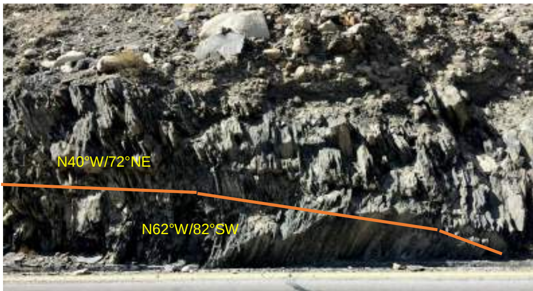
Photo 6-8 Change of Dip along Shear joint.
