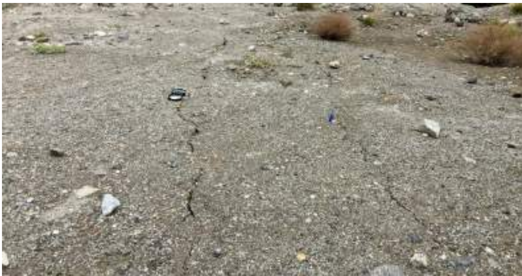
Photo 6-20 Development of Parallel Joints near SCO Building.
