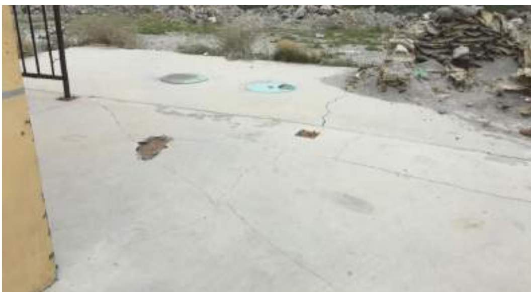
Photo 6-16 View of Recently Generated Joints Between Tunnel-2 & 3.
